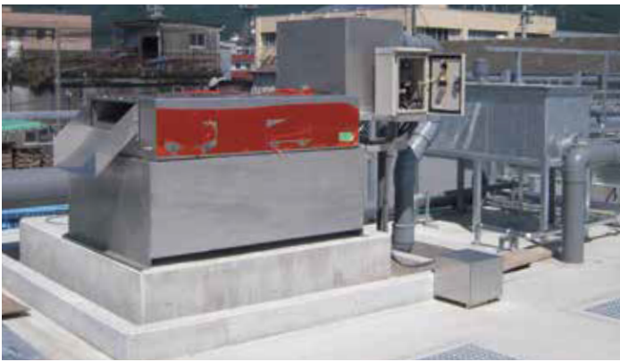
Marine product processing wastewater treatment
