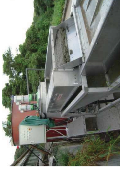
Pig dung wastewater treatment
